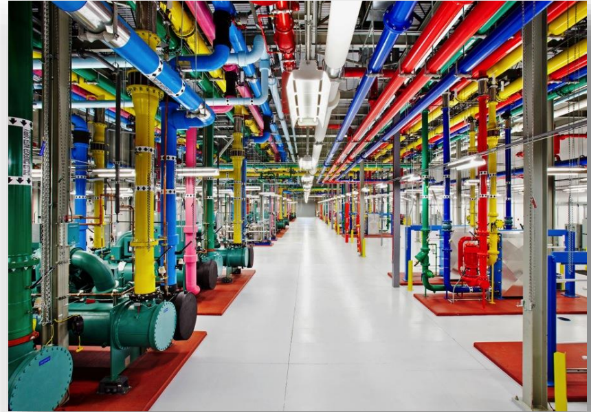
A central cooling plant in Google's Douglas County, Georgia data center.
